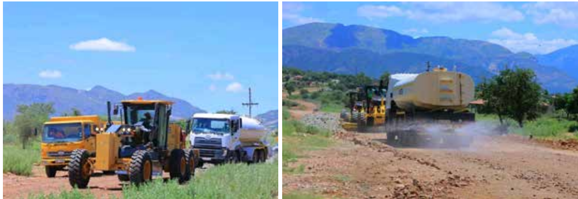
The Dikgerekgere service delivery initiative team rehabilitating dilapidated roads affecting four villages of Fetakgomo-Tubatse Municipality.
